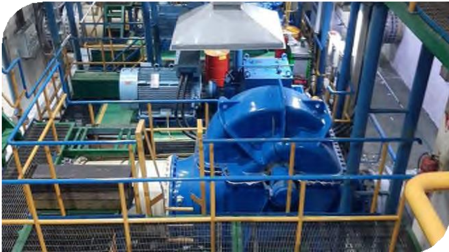
Maintenance Pump House Jasa Tirta - Cawang
